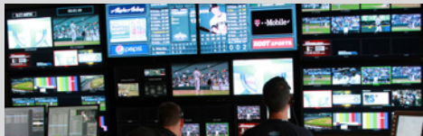
BROADCAST CONTROL ROOMS
